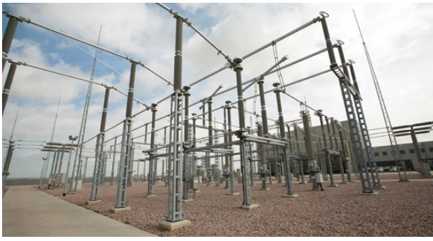
Figure 7: BritNed CSC converter station
